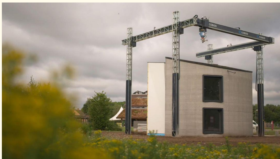
Figure 4: Europe's first 3D-printed two-story house in Belgium, alongside the BOD2 printer that created it.
