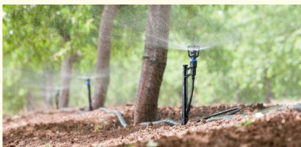
Figure 23 - Micro-sprinkler system (Campezza, n.d.)
